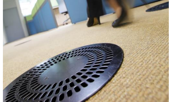
Gambar 34: Lantai difuser (Sumber: Architizer, 2024)
